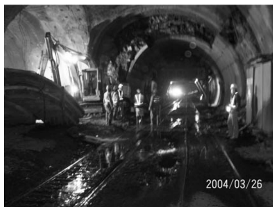
Figure.10 Water pipe lines, tracks...damaged
